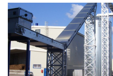
Material Handling Conveyor
