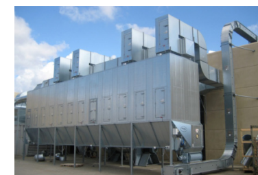
Conveying Blower to Silo
