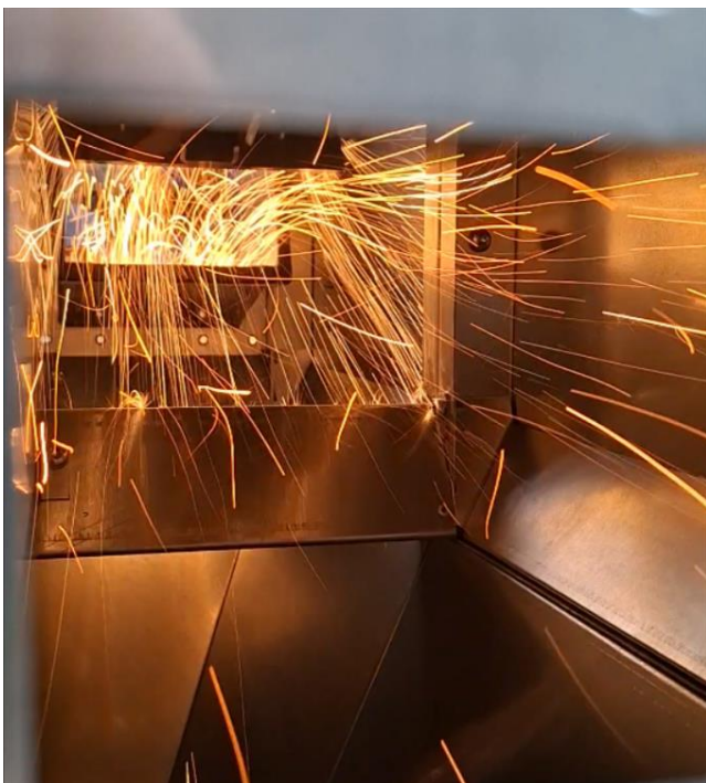
Inside the dust collector without spark screen
